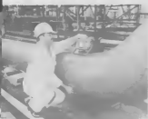
Inspector A.R. Valasquez ultrasonically (UT) checking the wall thickness of 24" pipeline at PS-5. The instrument in use is USM-2 Kraut-ramer.
